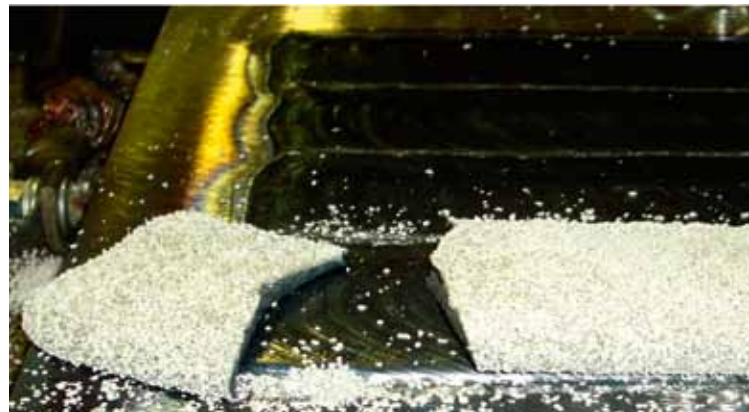
Full weld bead cladded with OK Flux 10.31/OK Band 7018). ESAB A6 head, 2 x ESAB LAF 1600 DC, PEH control unit. 1000A / 30V / 13 cm/min, DC+. All welds are free of surface defects.
