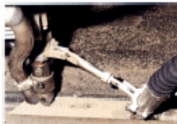
Figure 4: A6-S automatic welding machine during night-time operation. Flux-cored wire OK Tubrodur 15.65 (2.8 mm). Flux: OK Flux 10.62.
