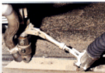
Figure 5: Top view of the build-up welded grooved rails. The beads display an even seam with smooth transitions. The layers approximate the final contour wherever possible, so that a minimum of grinding work is required.
