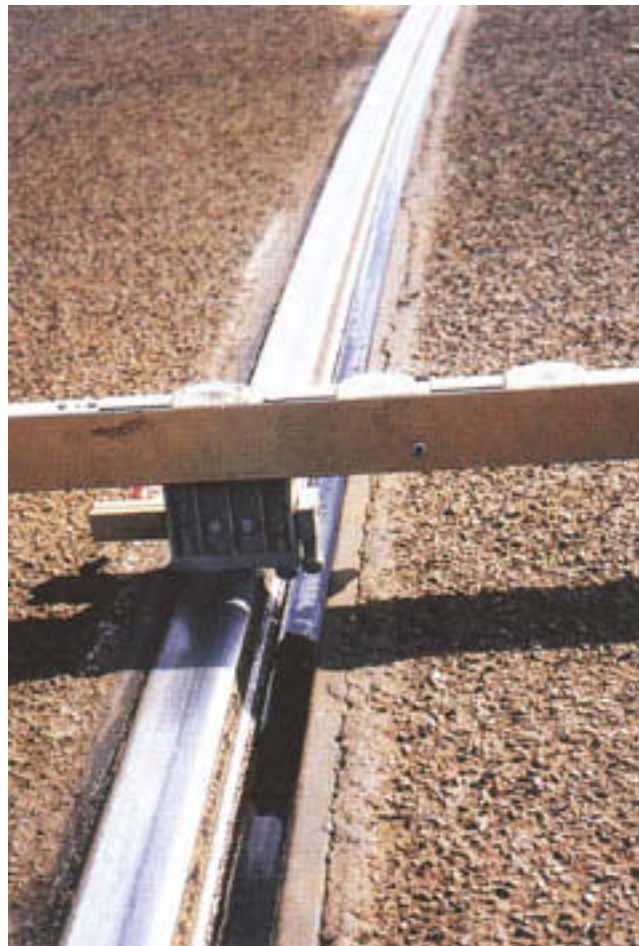
Figure 1: Introduction of the automatic welding machine in the track area or removal, during interruptions due to a tram passing
